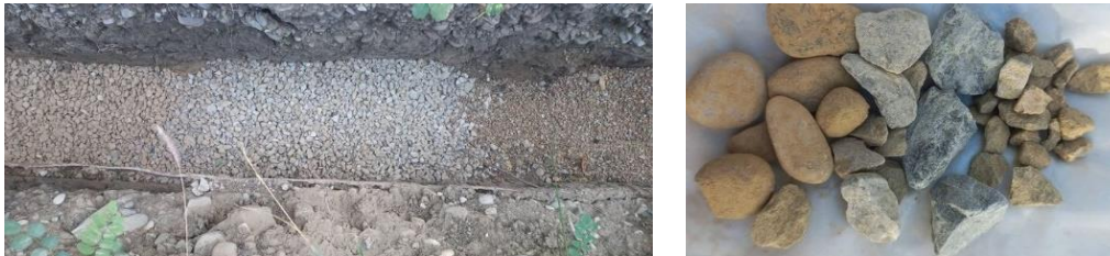
a) b) Figure 4. Aspects of laying a PE100 polyethylene pipe in a trench: a) pipe bedding; b) backfill material
