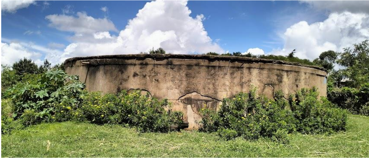
Figure 6: Water storage tank at Mua Hills. Source: Author 1 2024.
