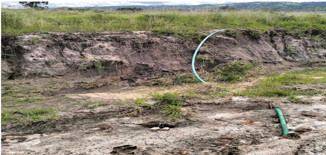
Figure 7: A vandalized water pipe in a Mua Hill settlement. Source: Author 1 2024.
