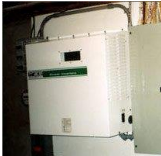
Figure-4: An Inverter (Source: US DoE)
